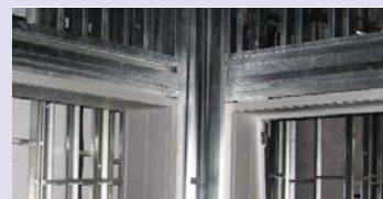
This complex sill and lintel system was recently installed around a window opening in an acoustic chase wall in a media studio.
