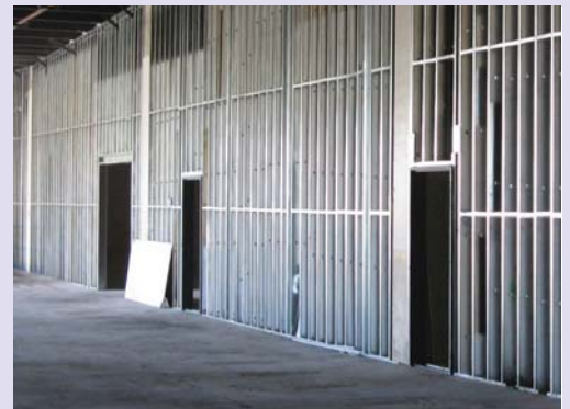
So many openings, so little information about how it should be constructed.
